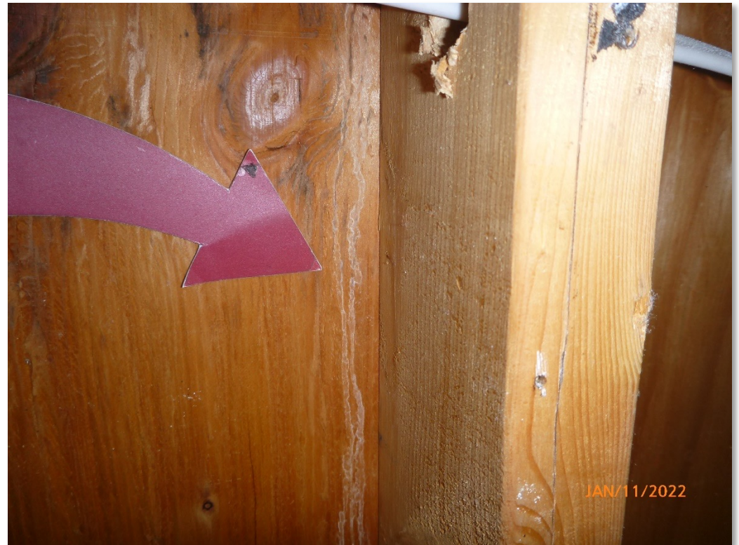
Water Intrusion from Roof Leak
