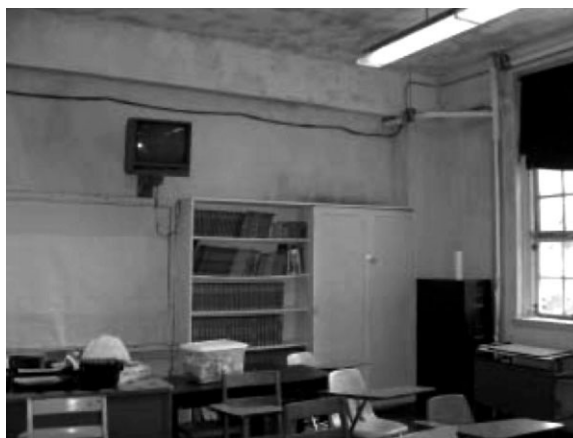
FIGURE 2. Picture of classroom wall and ceiling showing active mold growth at the water-damaged school.
